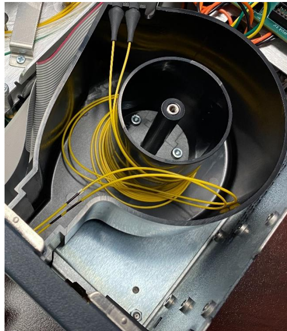
Figure 18: Exposed view of poor output fiber management
